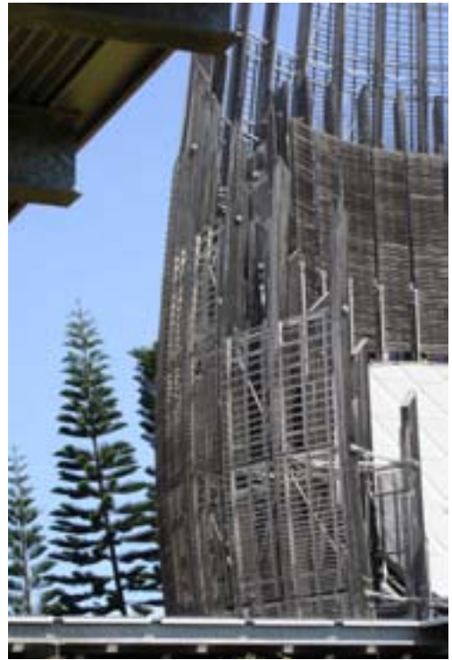
Figure 7. Steel frame underlying the fading iroko timber photograph by K Message, courtesy ADCK-Culturel Centre Tjibaou/ Renzo Piano Building Workshop, Architectes
